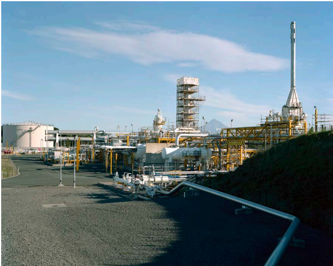
Pohokura Production Station #2, Motunui, 18th April 2012
