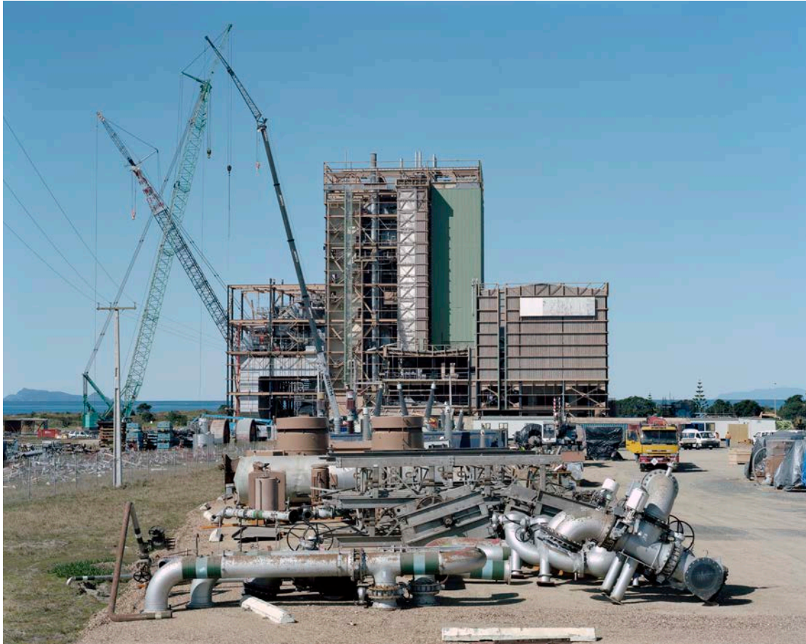
Marsden B Power Station in the process of being dismantled, Marsden Point, 27th August 2011
